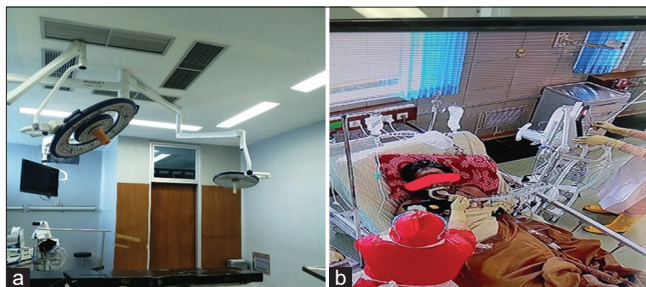
Figure 5: (a and b) Operating Room and ICU Isolation with the negative pressure
